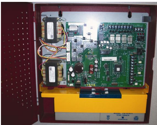
FCPS-24FS6 Remote Power Supply with yellow seismic battery bracket installed
