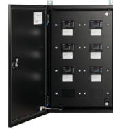
Multiple Meter Units (MMUs)
