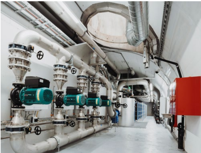
Alternately switched pumps for sustainable cooling with lake water
